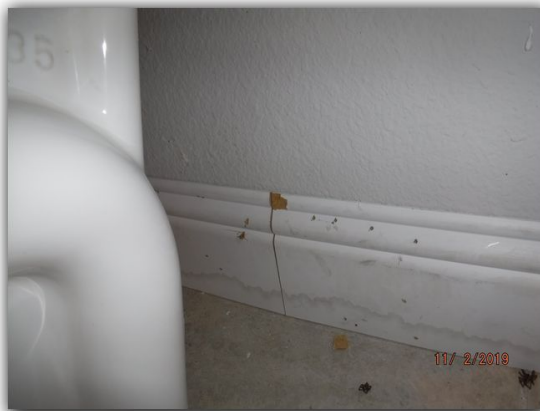
There is a hole above the electrical plate in the master commode room
