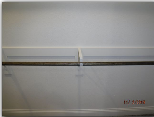
The baseboard behind the master commode needs attention
