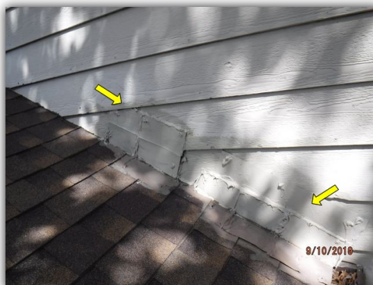
Going further up the same wall, more damage is seen. This siding is hardboard, which is easy vulnerable to damage from rodents. Recommend replacement with cement board
