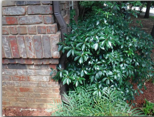
1/32 inch crack from center bottom of kitchen window to the foundation
