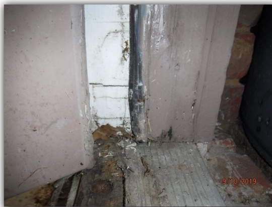
The back door weather stripping is worn
